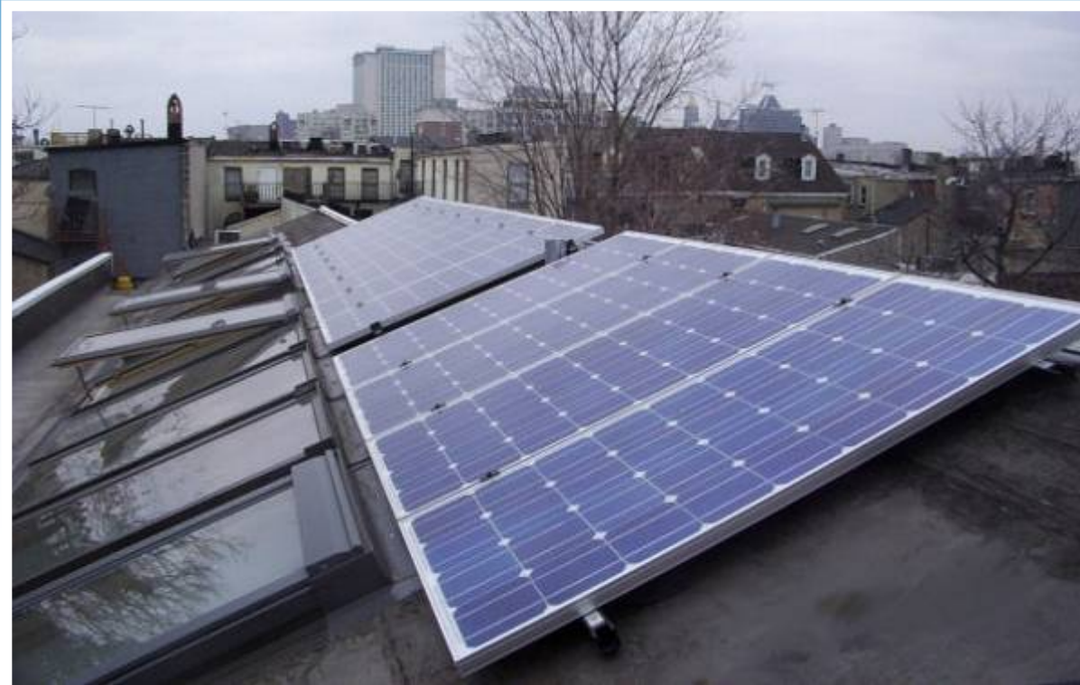
1.4 kW PV panel in Baltimore City (Source: Maryland Energy Administration)
